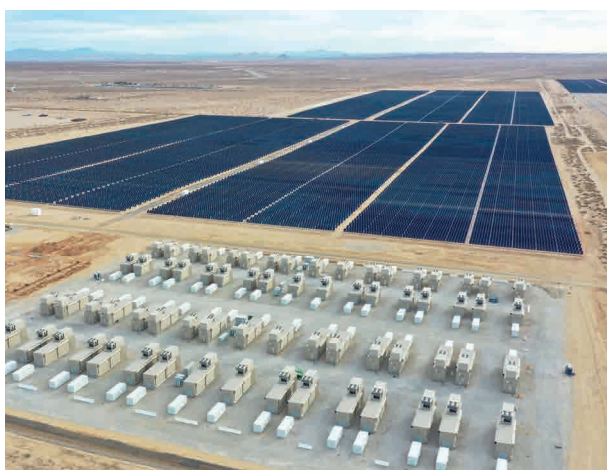
Edwards Sanborn Solar Storage Facility: the California project is the largest single solar and battery energy storage project of its kind
